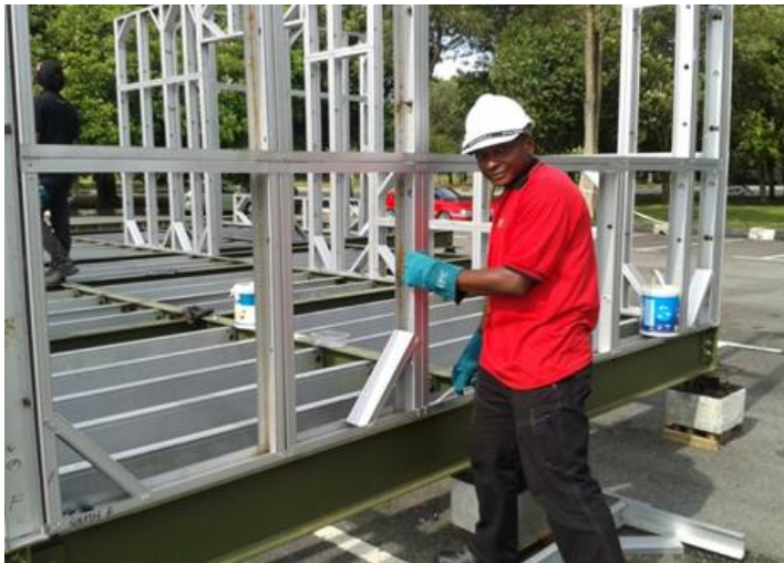
Figure 3 sample metal use for constructing wall frame to receive timber and wood members: Source authors' photo
